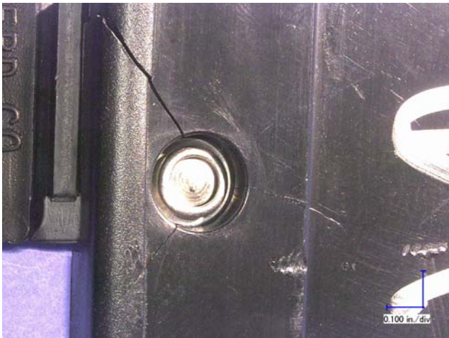
Fig. 8 - Cracks were present adjacent to the door hinges. The cracking shows no signs of significant macro ductility.
