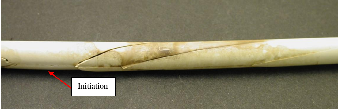
Figure 9: View of a freezing failure of a CPVC pipe in a residential setting.
