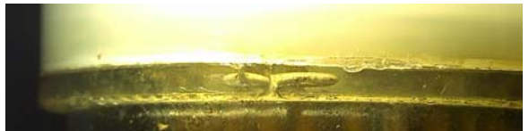
Figure 1: Pressure testing revealing the leak location and view of the failure location.
